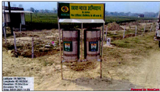
Figure 4: Installed steels dustbins for (wet and dry waste)
